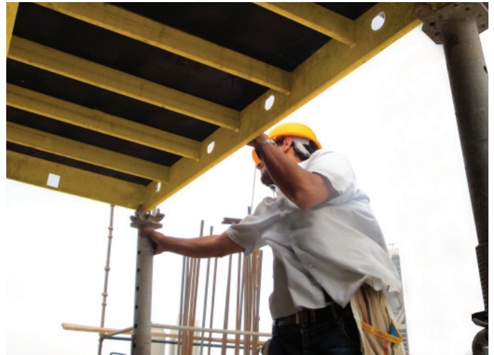
D. Final safety check to see that the panels are properly resting and fixed on the Top Deck Bearing.
