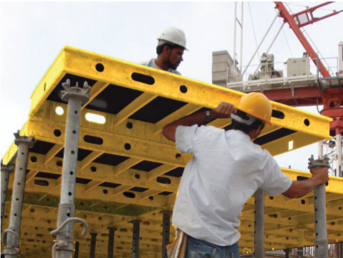
C. Final arrangement of the Alu Top Deck panels with clear positioning of the support in the corner of the panels.
