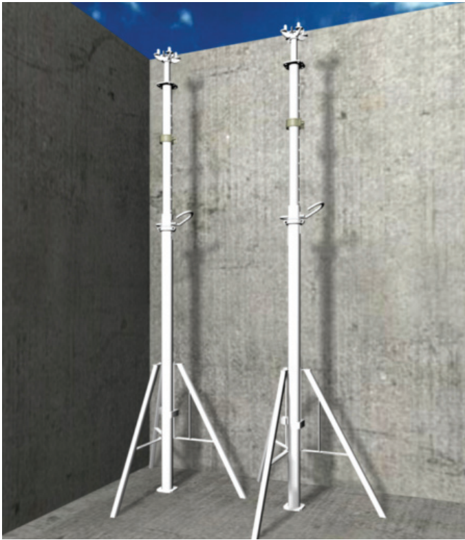
A. Position two steel props including Top Deck Bearing in the corner of the room with a distance of 90 cm and align vertically by means of Tripod Stand.
